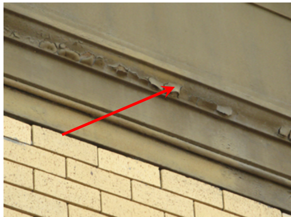
Figure 61. Delaminating paint. Source: Page & Turnbull, March 2010.
