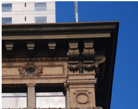
Figure 64. Area of exposed sheet metal with no paint. Source: Page & Turnbull, March 2010.
