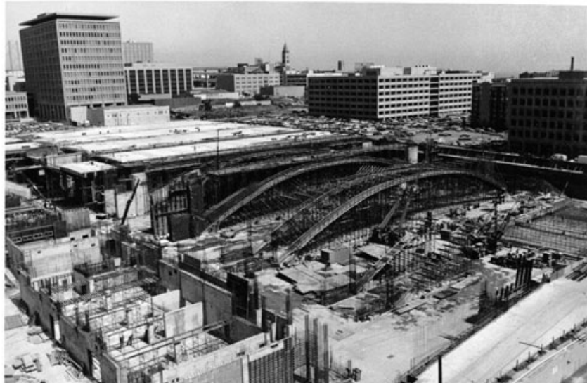
Figure 05. Construction of Moscone Convention Center, 1980. Source: San Francisco Historical Photograph Collection, AAC-0724.
