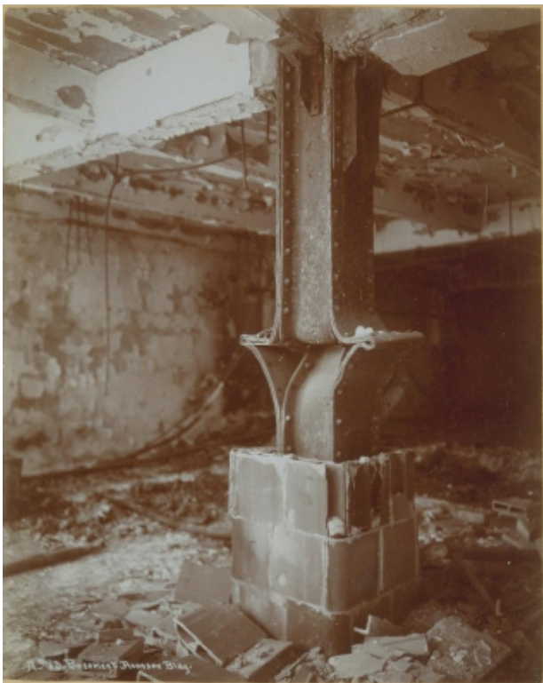
Figure 13. Buckled I-beam encased in failed hollow tiles in the basement, 1906. Source: Bancroft Library.
