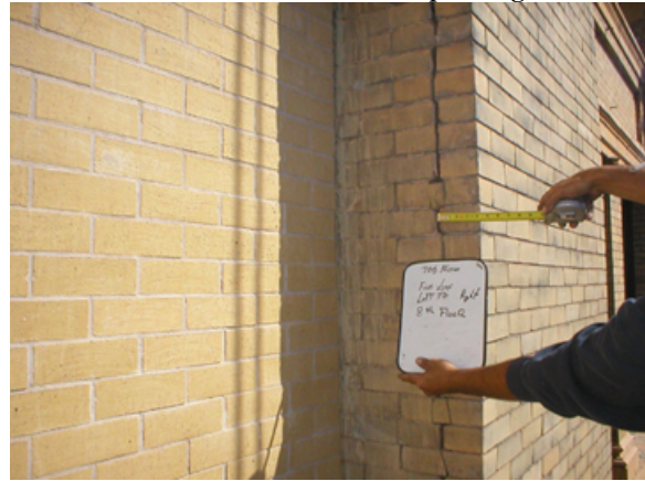
Figure 51. Cracking of terra cotta brick. Source: Rainbow Waterproofing, 2006.
