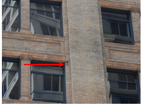
Figure 59. Missing brick. Source: Page & Turnbull, March 2010.
