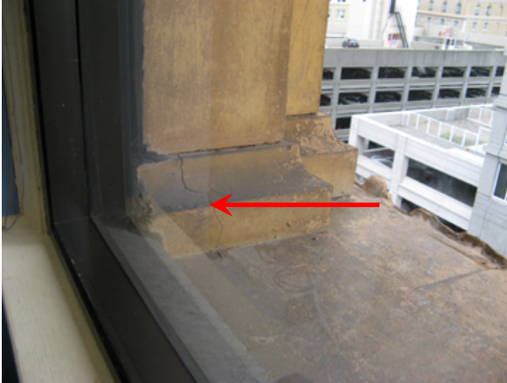
Figure 54. Cracking at column base. Source: Page & Turnbull, March 2010.
