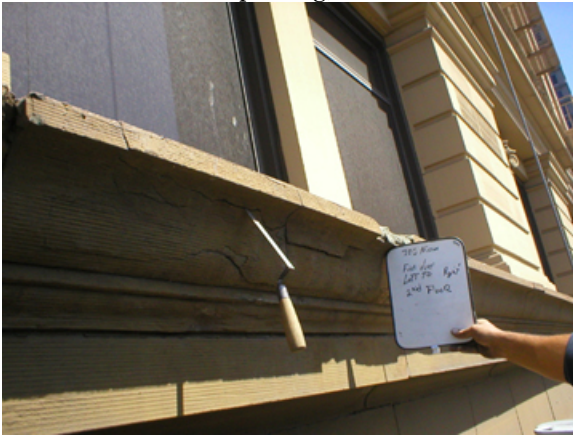
Figure 50. Cracking of sandstone. Source: Rainbow Waterproofing, 2006.
