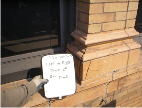
Figure 46. Cracking at column base. Source: Rainbow Waterproofing, 2006.
