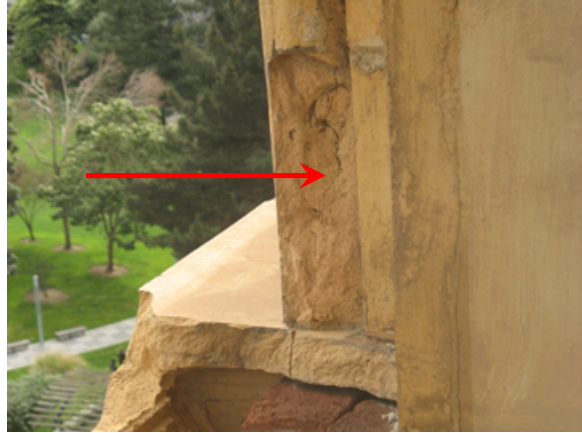
Figure 55. In-plane cracking at bisque spall. Source: Page & Turnbull, March 2010.
