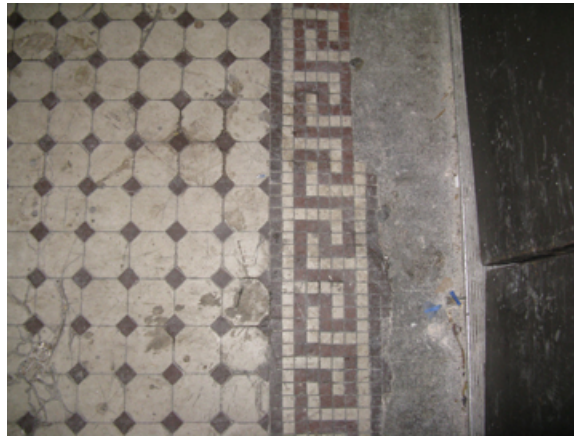
Figure 67. Cracking and soiling of ceramic tile. Source: Page & Turnbull, March 2010.
