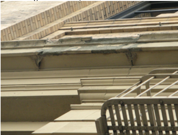
Figure 41. Spalling of sandstone at edge. Source: Page & Turnbull, March 2010.
