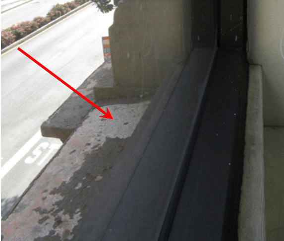
Figure 62. Area of exposed cast iron with no paint. Source: Page & Turnbull, March 2010.
