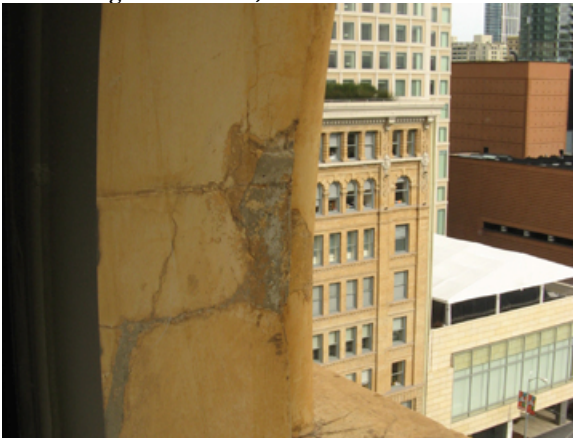
Figure 56. Previous repair. Source: Page & Turnbull, March 2010.
