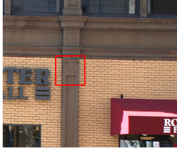
Figure 63. Missing scroll at column capital on 3 rd Street facade. Source: Page & Turnbull, March 2010.
