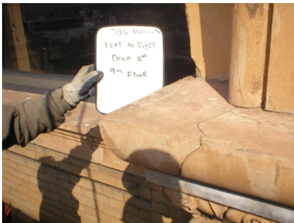
Figure 44. Cracking at cornice. Source: Rainbow Waterproofing, 2006.
