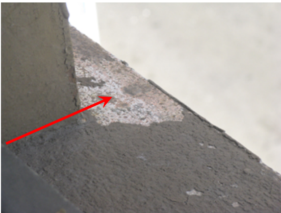
Figure 60. Corrosion of cast iron. Source: Page & Turnbull, March 2010.
