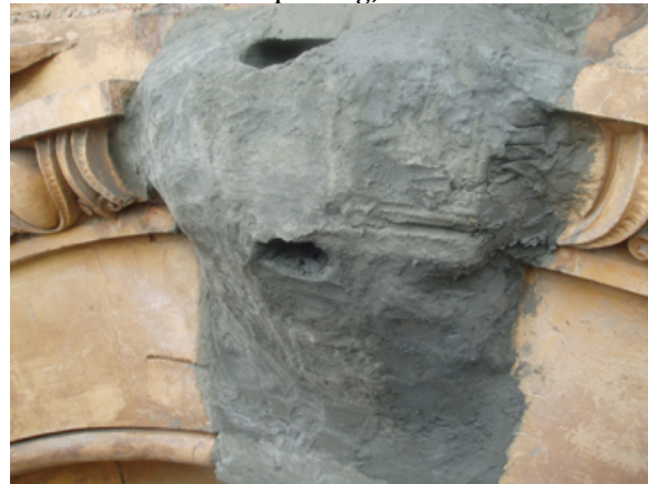
Figure 49. Removal of cracked and mortar patch of piece shown at left. Source: Rainbow Waterproofing, 2006.
