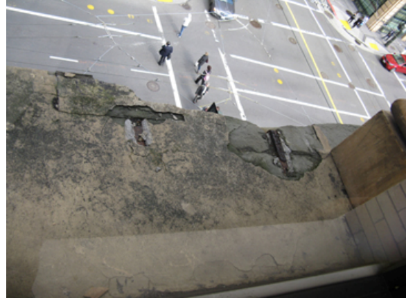
Figure 40. Cracking/spalling of concrete at steel corrosion. Source: Page & Turnbull, March 2010.
