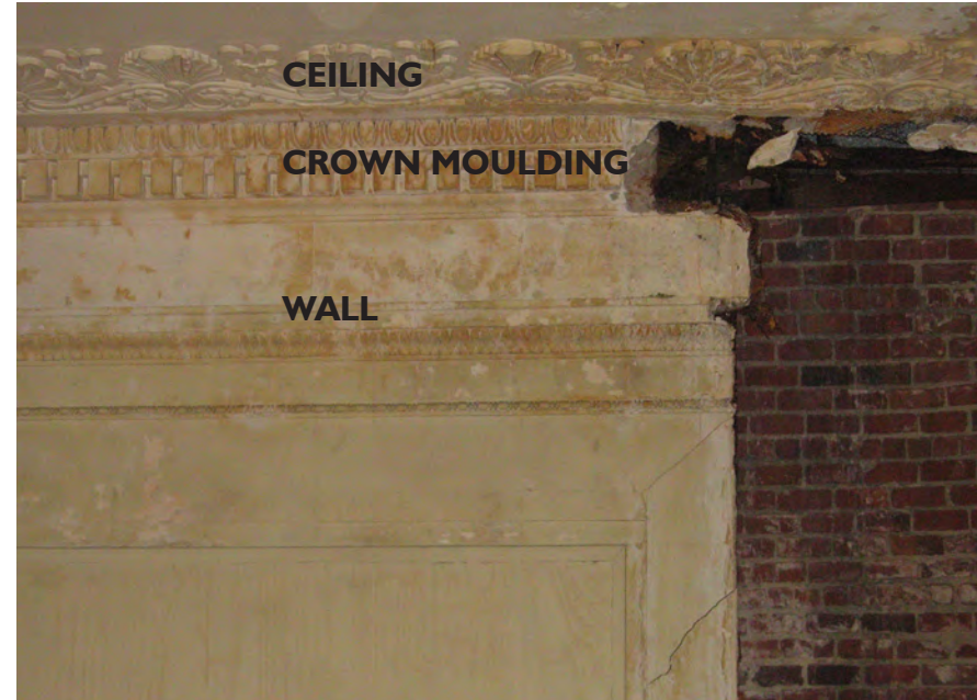
Deteriorated plaster where wall meets ceiling
