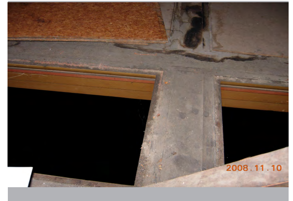
Close up view of wood laylight showing area where glass panels are missing
