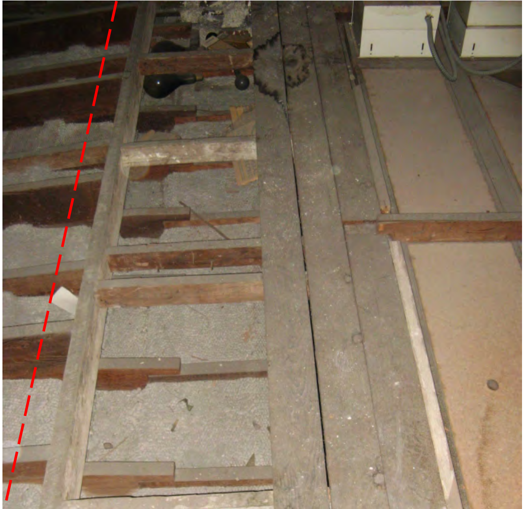
Figure 8: Framing above Exchange Hall ceiling, north of the north west corner laylight, showing cut line (red line) outside of underlying beam, approximately four feet from the laylight. This cut should be continued on the west side of the laylight.
