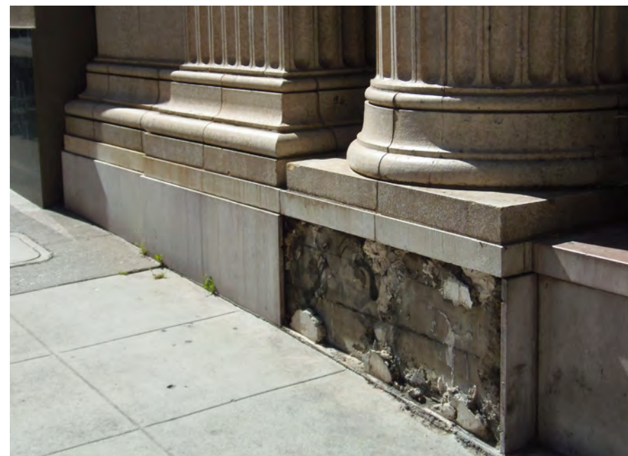
Missing stone panel will be replaced in kind
