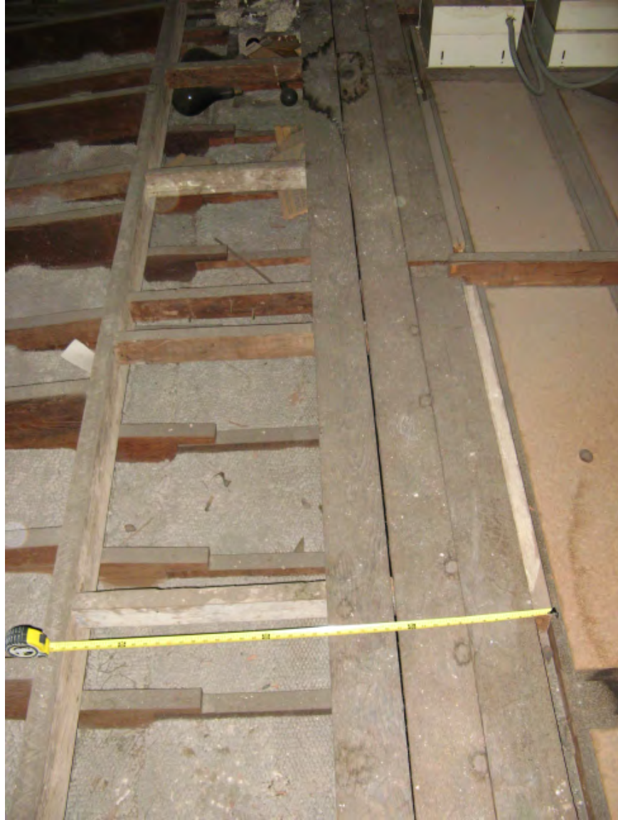
Figure 6: Framing above Exchange Hall ceiling, north of the north west corner laylight, showing top of laylight (right), walkway (center), and formed metal lath covered with plaster which forms the panelled beams below (left). The plaster and lath is nailed to wooden joists and filler pieces.
