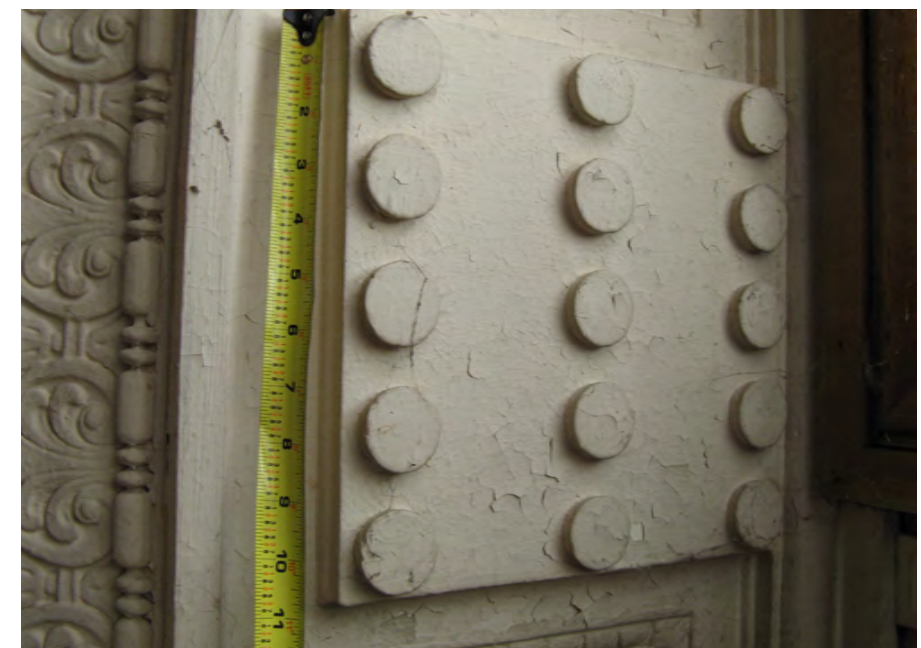
Deteriorated Plaster Ceiling and Cornice detail
