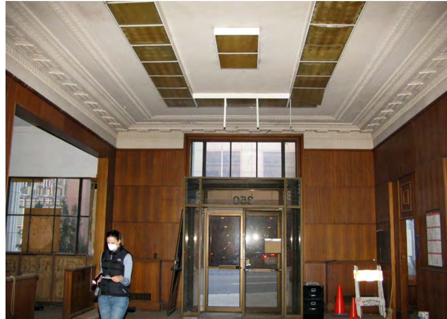
Entry Hall looking south. Note that a portion of the ceiling was removed when the aluminum doors were installed
