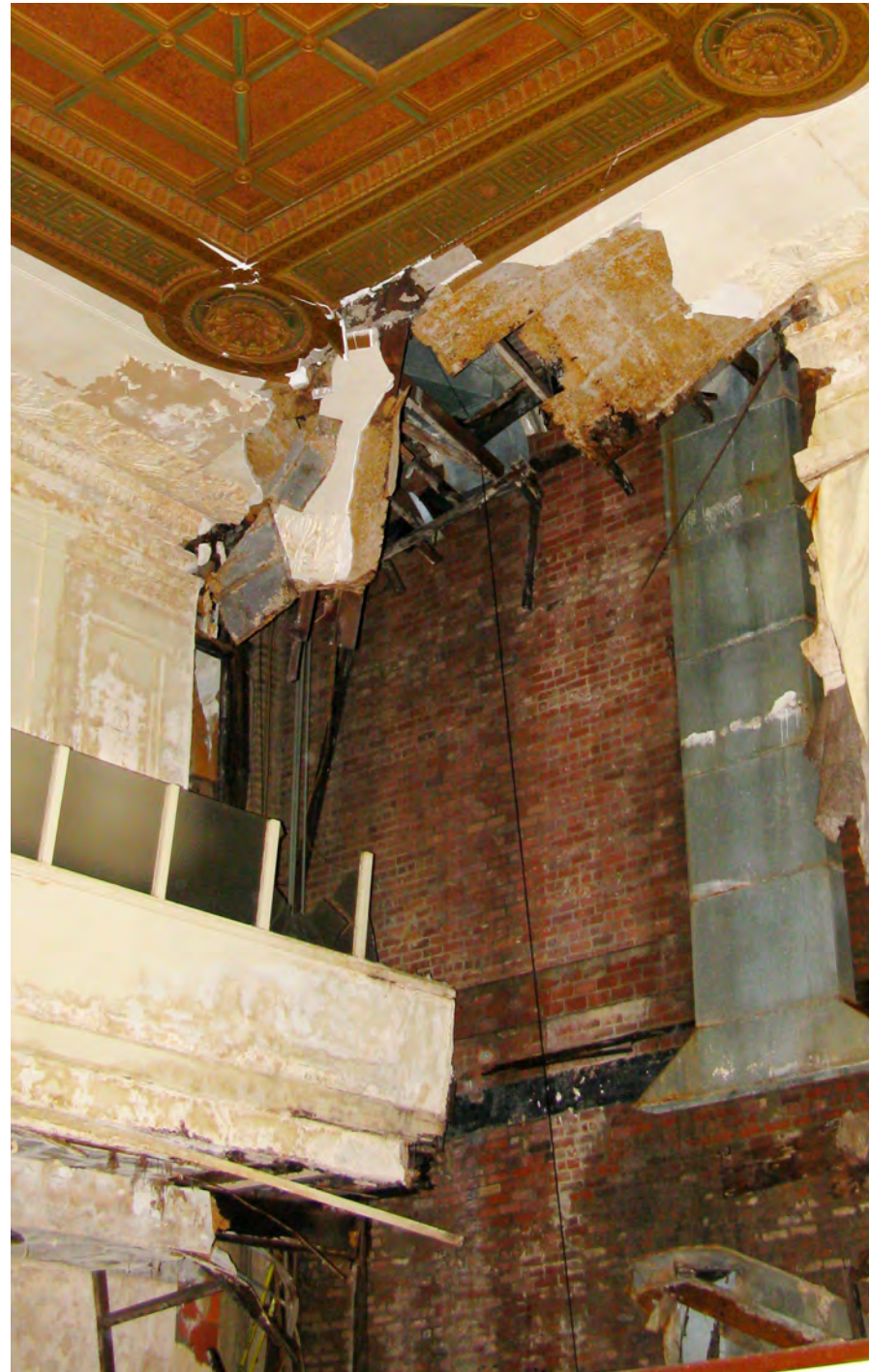
Deteriorated Plaster Ceiling and Cornice and wall detail
