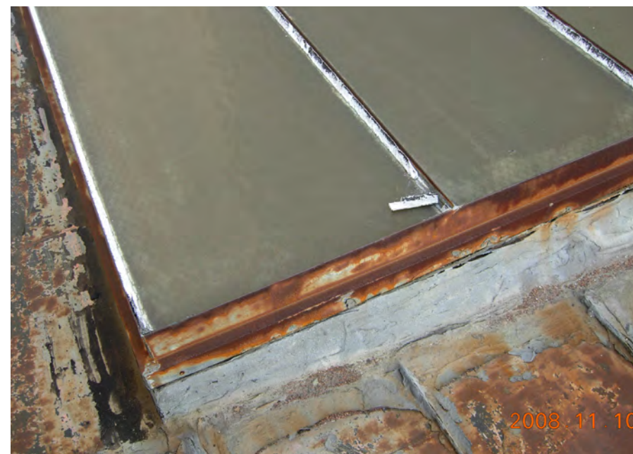
Galvanized steel skylight with wire glass exhibiting deterioration
