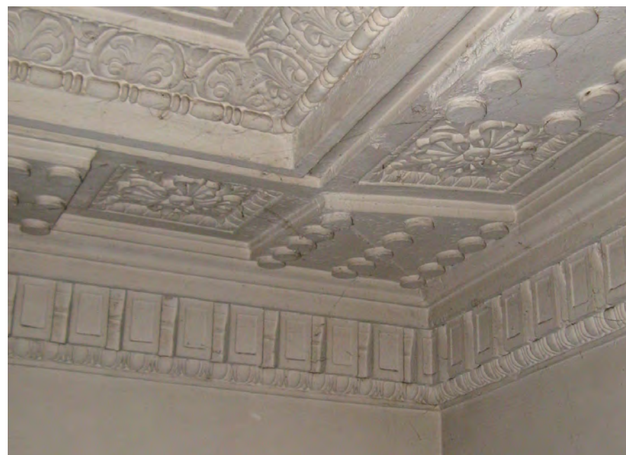
Deteriorated Plaster Ceiling and Cornice detail
