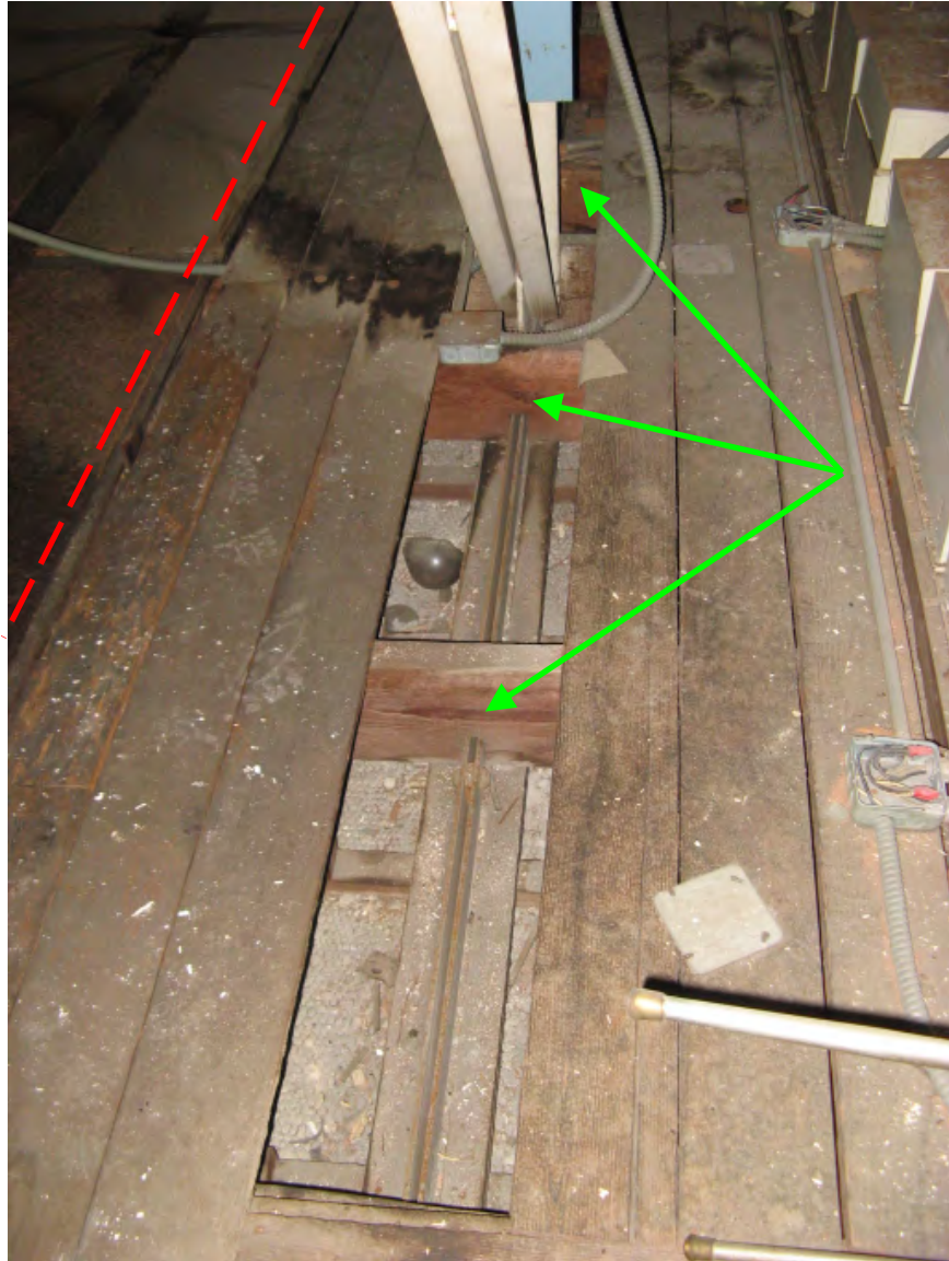
Figure 9: Framing between north west laylight and adjacent laylight, showing walkway planks to be removed prior to cutting of framing and plaster. Also shown are joists to be cut (green arrows) and cut line of plaster and lath near adjacent laylight (red line). This should be repeated on the south side of the laylight.
