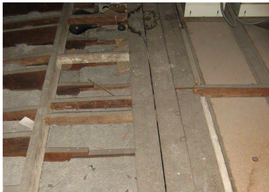
Above perimeter plaster molding where ceiling slopes down to crown Note: laylight and non-historic masonite on right side
