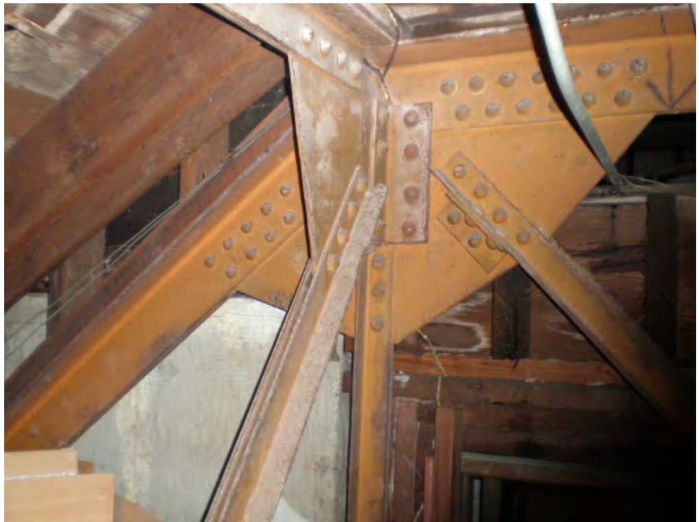
Figure 5: Attic above Exchange Hall ceiling, showing riveted steel frame that supports roof and laylights.
