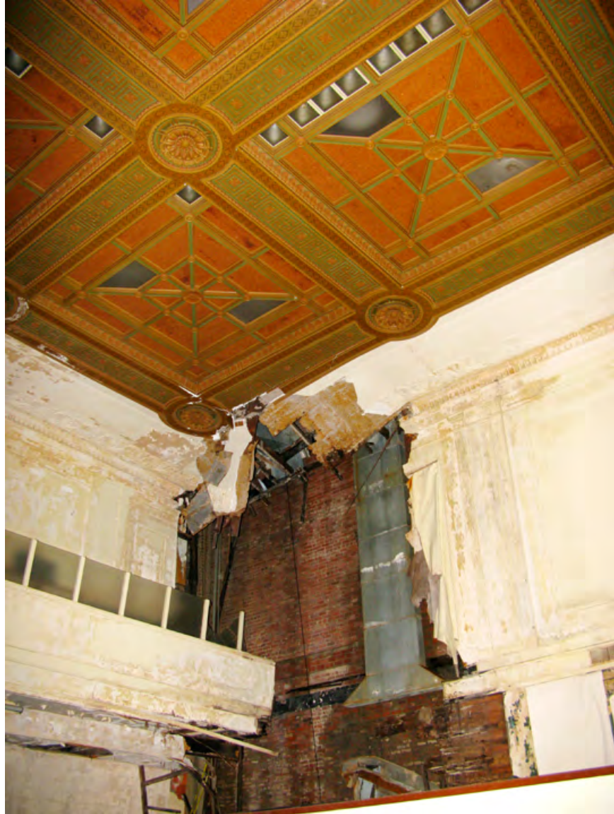
Figure 3: Loss of wall panels and part of the ceiling, southwest corner of Exchange Hall.
