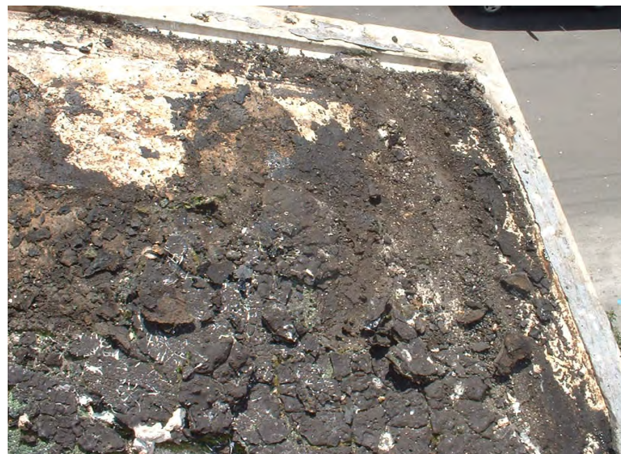
Existing photograph showing the top of the terra cotta raking cornice. The acroteria would have attached to the cornice.
