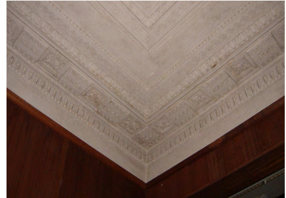
Deteriorated Plaster Ceiling and Cornice
