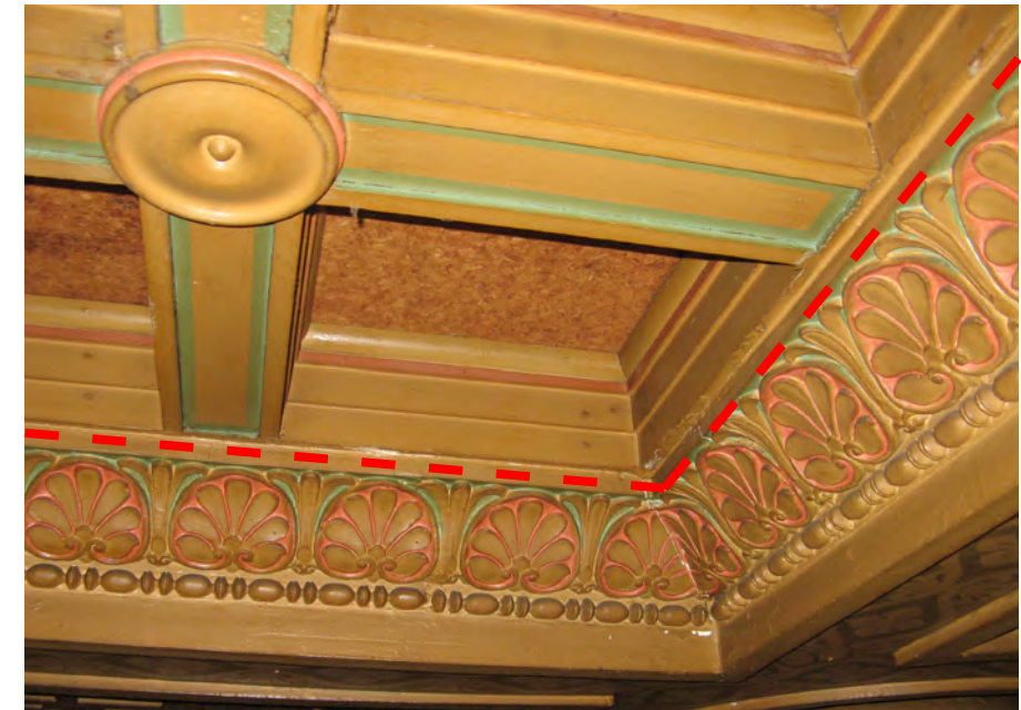
Wood Laylight Assembly to be salvaged for replacement Note: Dashed line indicates proposed area for removing laylight and plaster.
