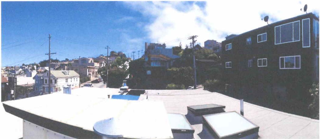
Roof of atrium and skylights to bathrooms and connecting hallway at 770 De Haro Street
