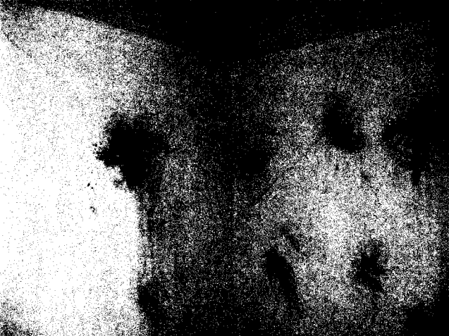
Photo 65: Cracks & Damages on Front Bedroom Wall
