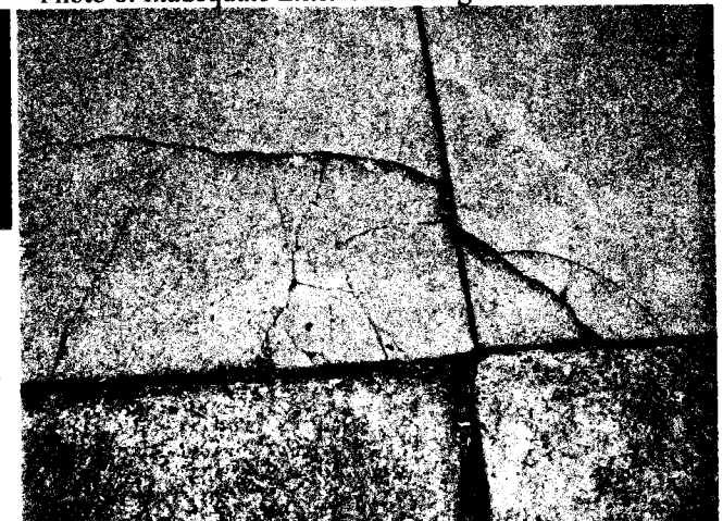
Photo 10: Damaged Driveway & Sidewalk Slab
