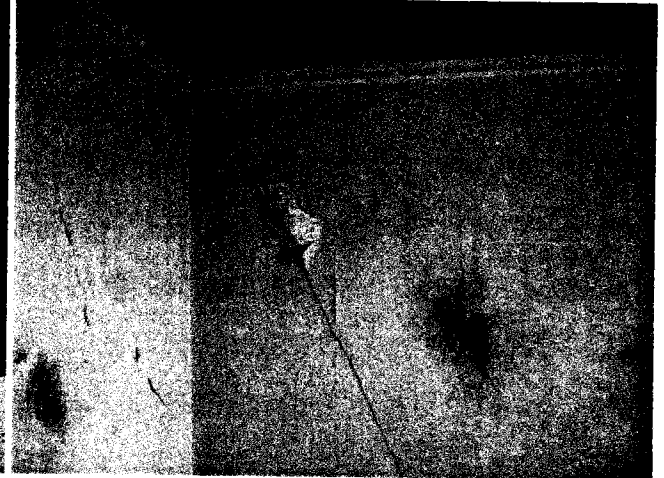
Photo 70: Damages & Cracks on Rear Bedroom Wall
