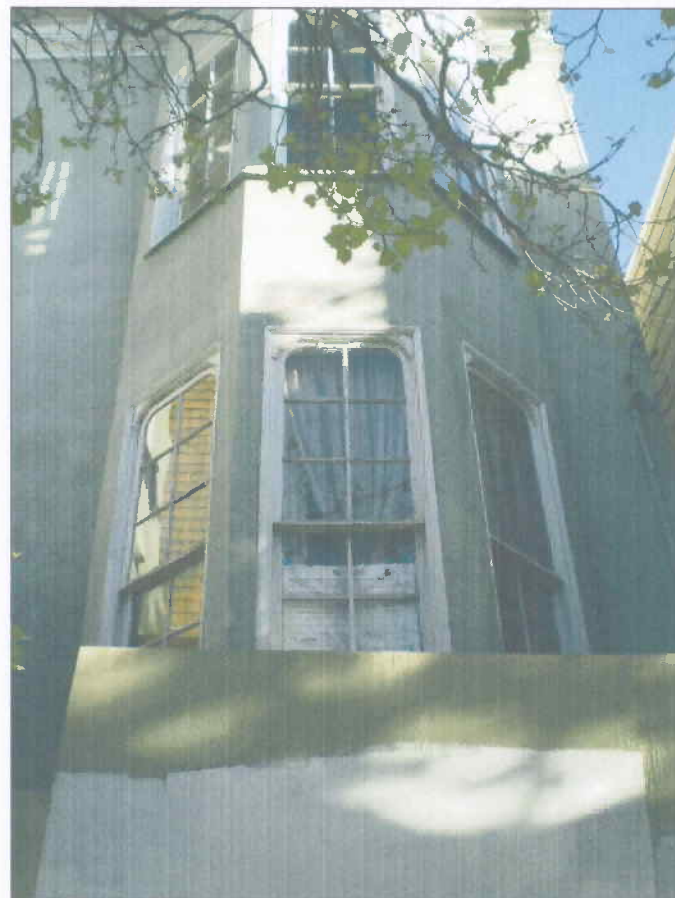
640-642 HAYES STREET FACADE WINDOWS
