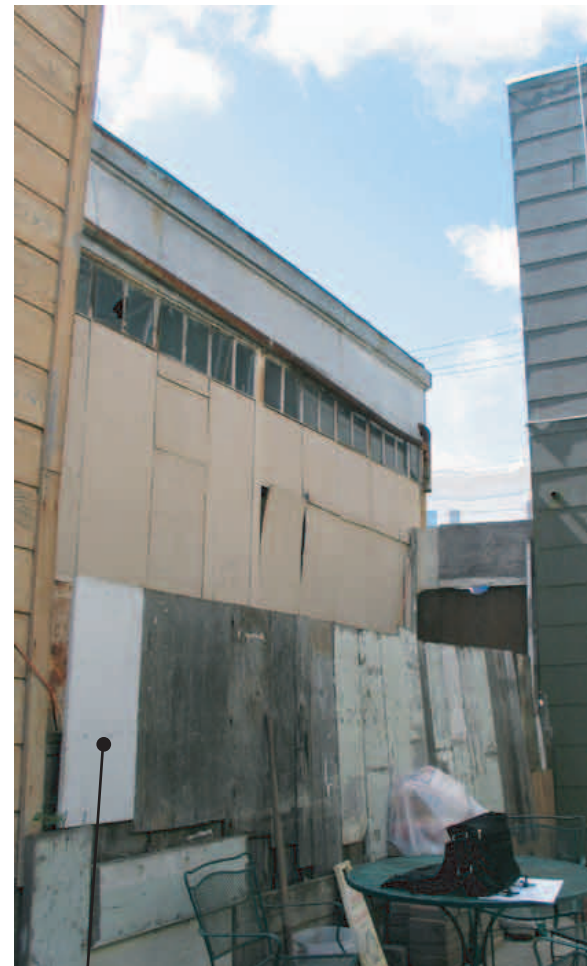
Fence to be repaired
