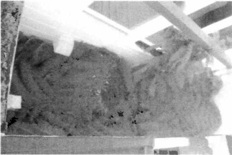
plants in the light well at 66 Rico blocking light to the windows below
