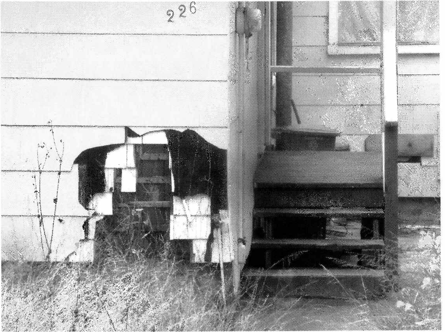
Close-up picture of green wood showing near foundation behind weeds. Picture taken July 2010
