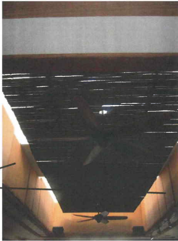
The Brick Yard skylights with sound panels on vertical walls covering approx. 500 sq ft
