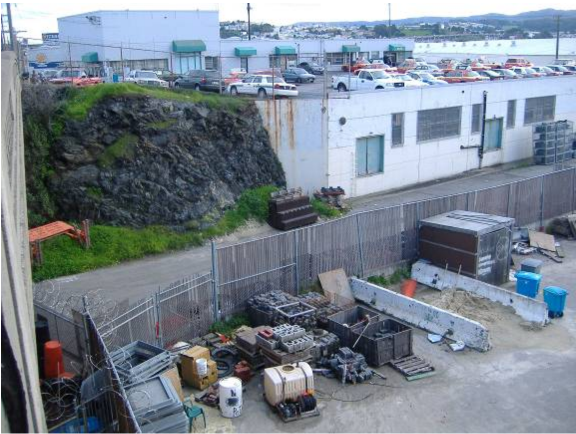
15 - View from Army street bridge looking back at 2121 Evans site to the SE - rock outcropping on left to stay, white building to be removed and new retaining wall built
