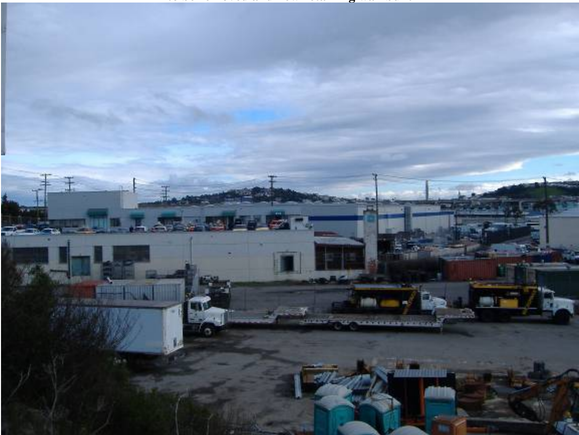
16 - View from Army street looking S toward 2121 building to be demo'd (green awnings) and RD building to remain (blue stripe)
