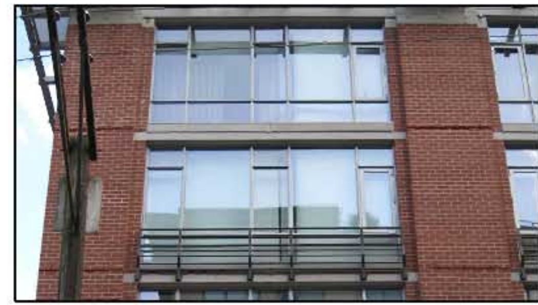
16 EXPOSED CONCRETE AT SLAB EDGE
