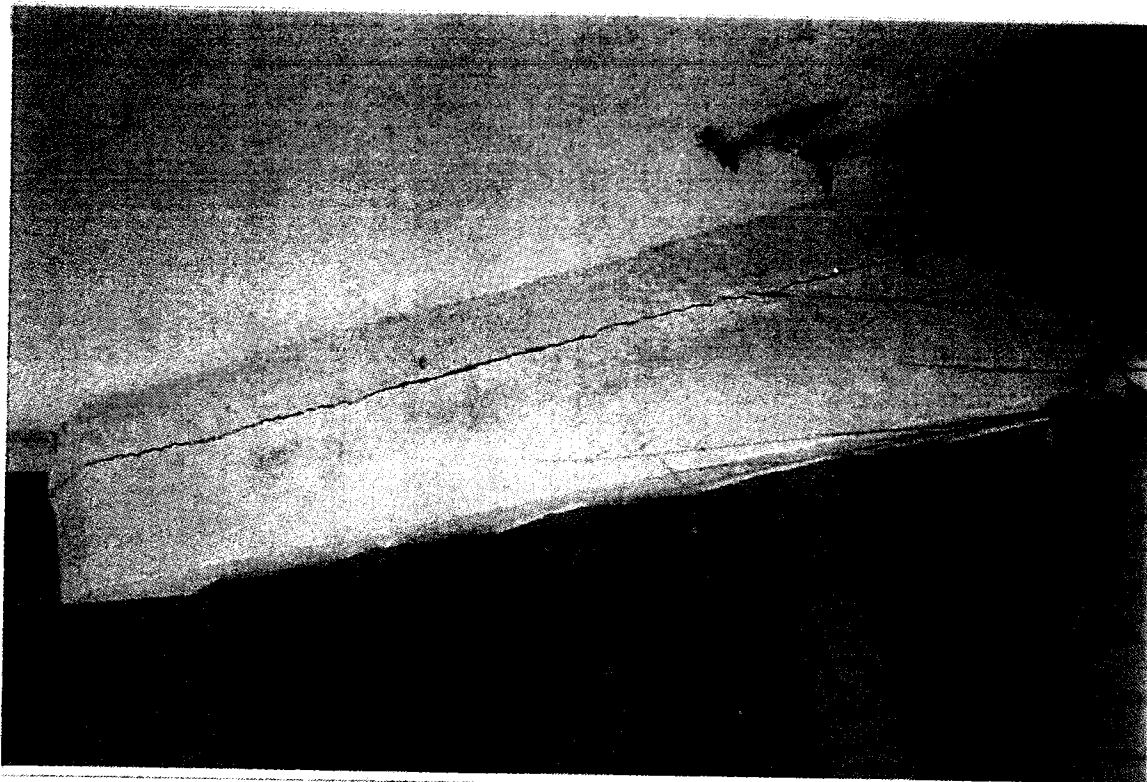
3. Front Stair Movement Due to Slide
