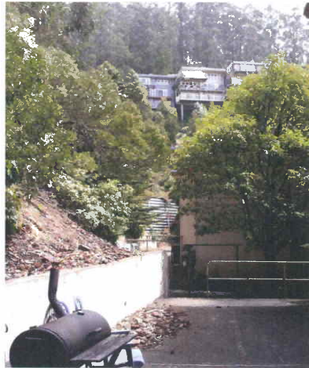
Picture #10: Debris falling over retaining wall into backyard (next to BBQ/smoker)
