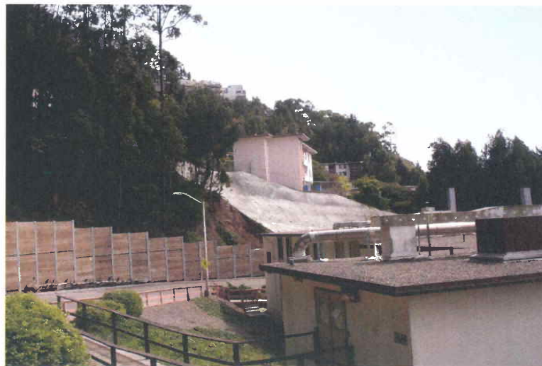
Picture #11: Retaining walls and concrete supported with rock bolts at base of Mt. Sutro
