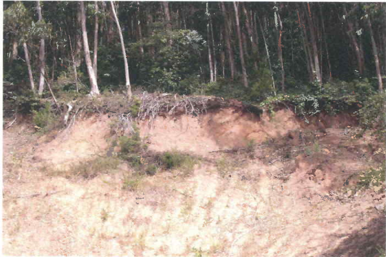
Picture #13: Existing erosion. Note exposed roots. Potential for mudslides with next heavy rain.
