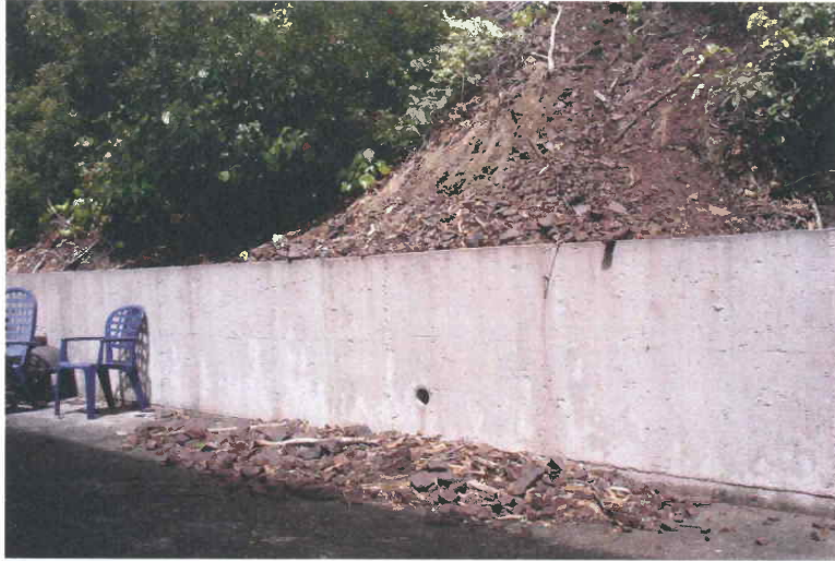
Picture #8: Debris flowing downhill behind Kirkham Heights building.
