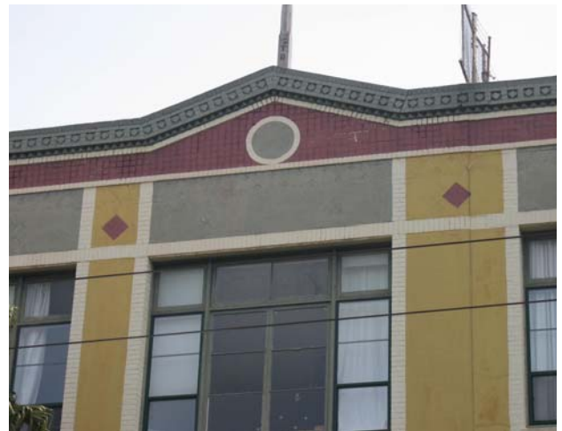
Façade, cornice, and parapet details of the Redlick-Newman Co. building. View east. The boundary between the original structure (left) and the southern addition (right) is visible as a vertical line that runs through the wider pilaster that is located right of center. San Francisco Planning Department.
