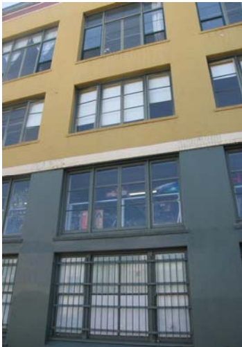
Bands of large divided metal-sash windows with brick water tables, located on the 17 th Street façade. View south. San Francisco Planning Department.
